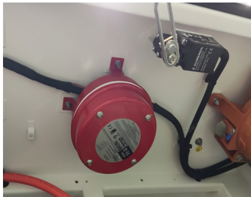
Figure 5-29 Aerosols activated by thermal sensitive wires
